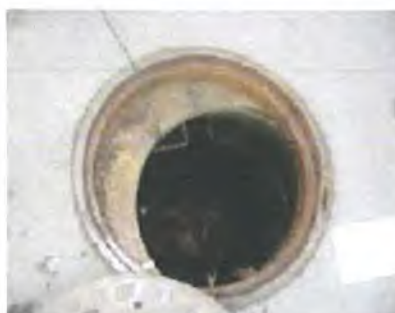
Figure 2: Offset of manhole block
