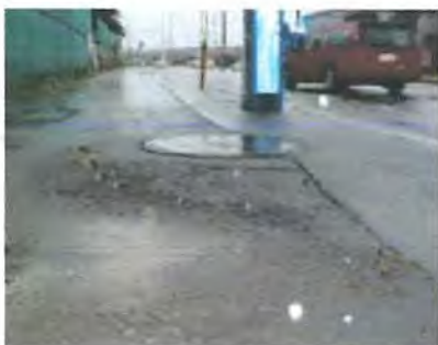
Figure 3: Not coinciding with height of road surface.
